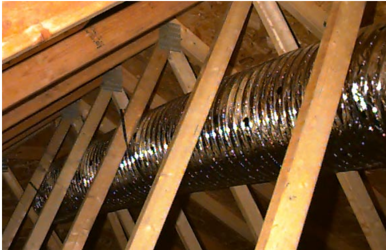
Perforate duct mounted near apex of attic.
