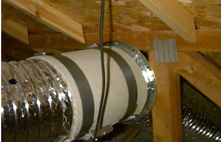
Ridge ventilator has an in-line blower assembly.
