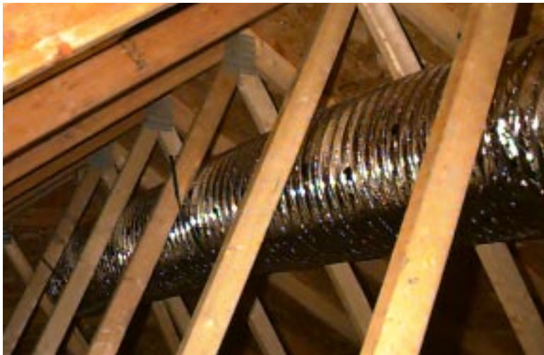
SolarAttic’s new duct technology at apex of attic.
